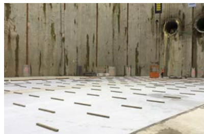
Pump Station Oberhausen | Germany
