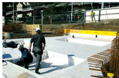
Residential Complex Bucheggplatz Zürich | Switzerland
