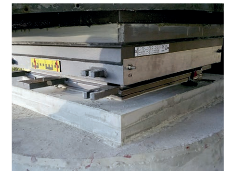
Pot bearings after installation
